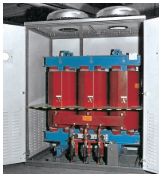
Fig. 54: GEAFOLE transformer in protective housing to IP 20/40
